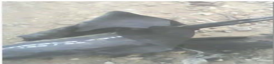
Figure 6. Faulted cable photograph before repairing
