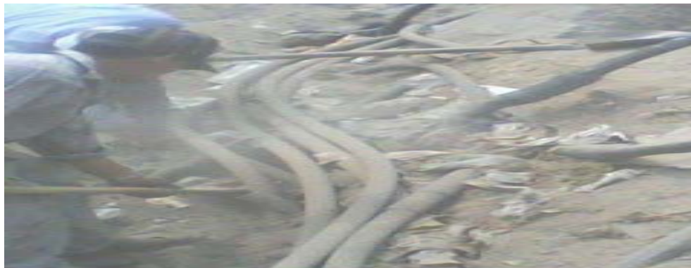
Figure 8. Faulted cable photograph before repairing
