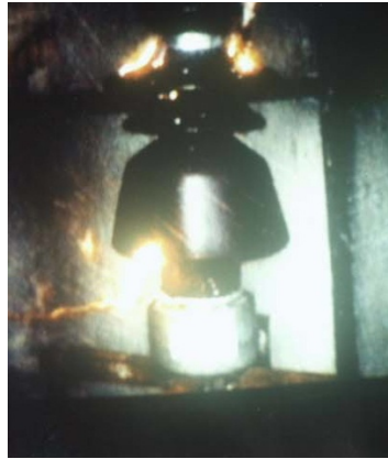
Figure 11. Flashover on the uncoated insulator
